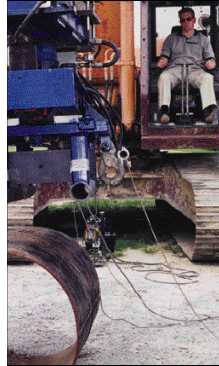
R. Kelly Barnhill, Jr., P.E., of the AGC firm Barnhill Contracting Co., Raleigh, N.C., tested an earlier prototype in the company's equipment yard. "All the field tests are so crucial for our research. I can't thank these contractors enough for their support," says Bernold.
