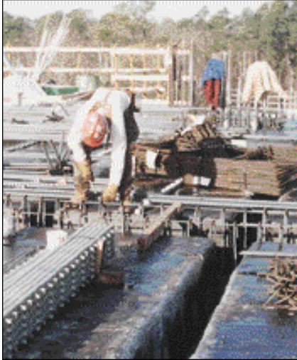
Intelligent rebar placement with planned rebar staging [for beam-joist floor] increased productivity 30 percent. Color taps on bundles show where to stage bar on formwork.
