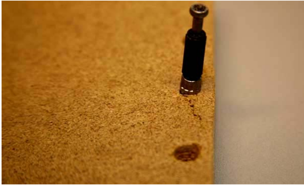
Fig. 12. The damage form of the connection with Rastex
