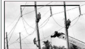
A Progress Energy crane moves away from power lines that it hit at Gorman Street near Western Boulevard. Staff Photo by John L. White
