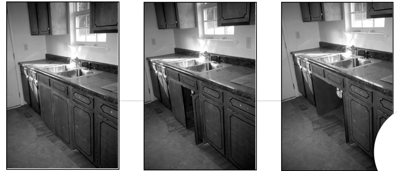
Swinging retractable cabinet door solution installed in a Habitat house during construction.
