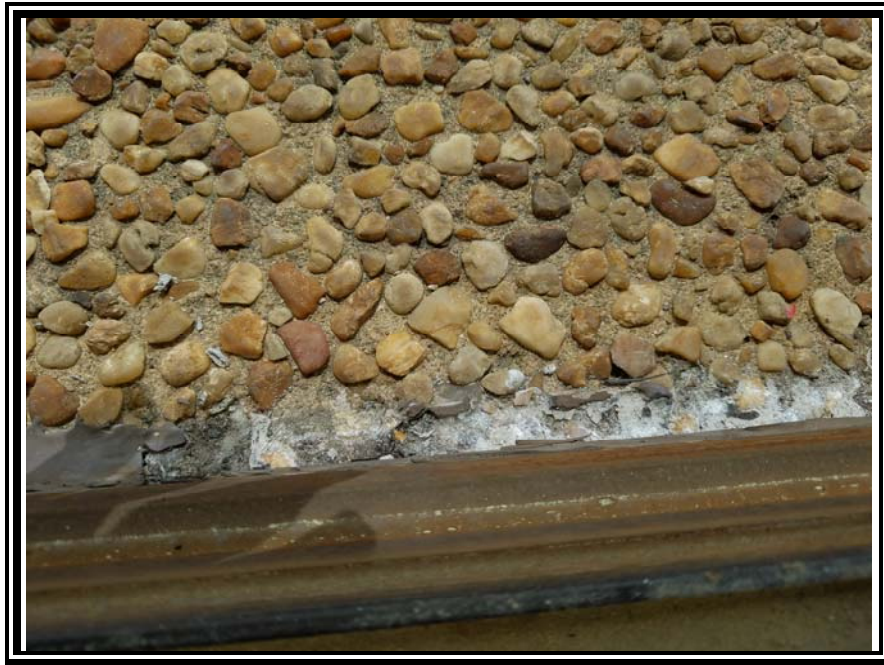
Poe Hall – POE-1 Window caulk with PCB's >50 PPM
