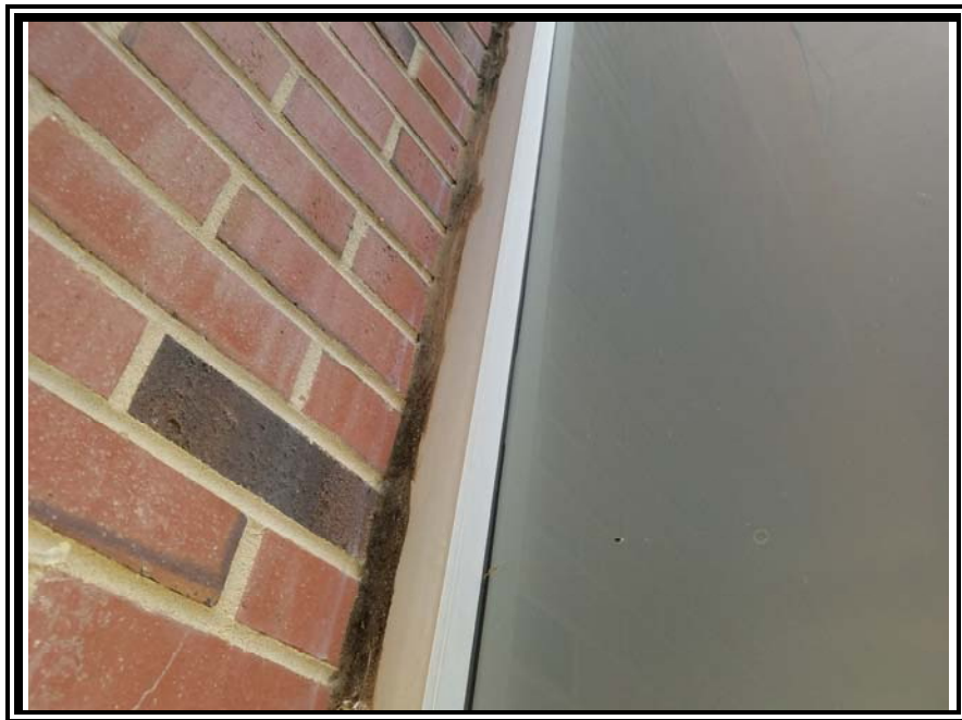
DH Hill Library – DH-2 Gray window caulk with PCB's >50 PPM
