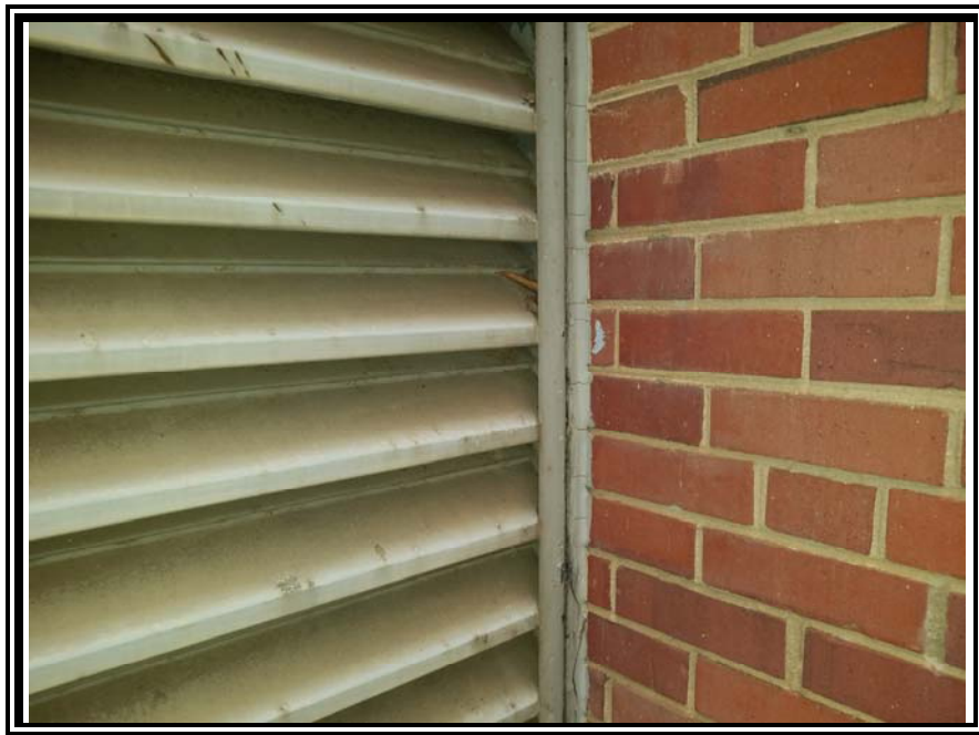
DH Hill Library – DH-4 Vent caulk with PCB's <50 PPM
