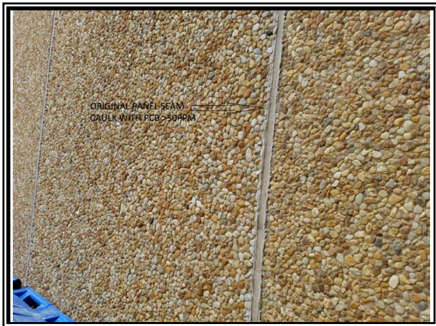
Poe Hall – POE-2 Panel caulk with PCB's >50 PPM
